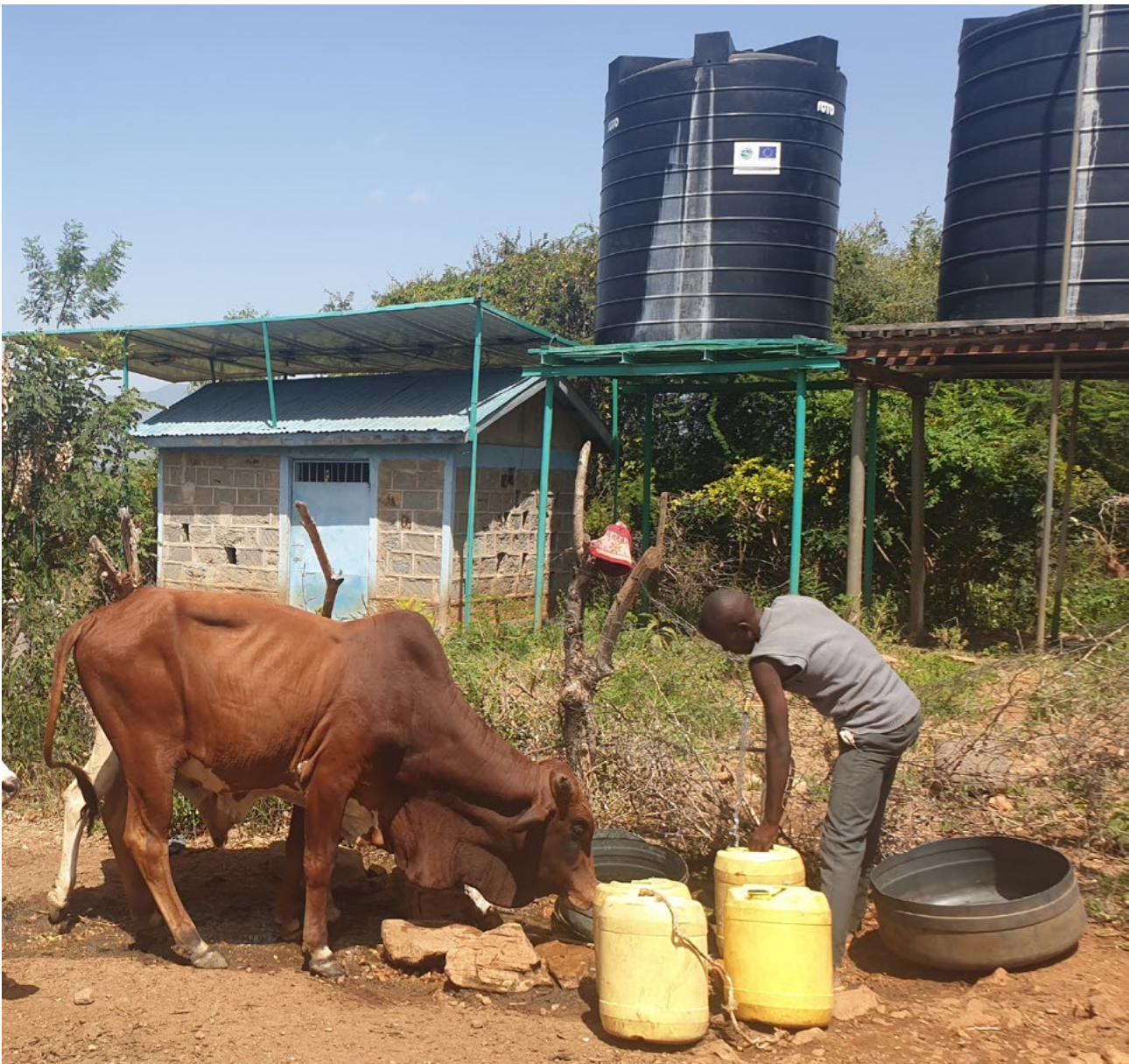
Solar panels installed at Cieria borehole.
